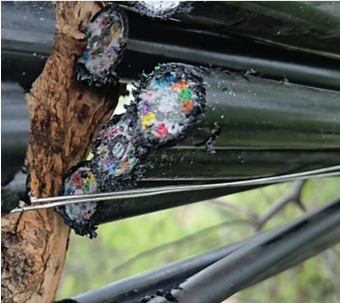
Spectrum Fiber optic lines were intentionally cut by a criminal attack that caused an outage to some customers in Sunland and parts of Tujunga and Sylmar. Spectrum fiber lines do not contain copper.
